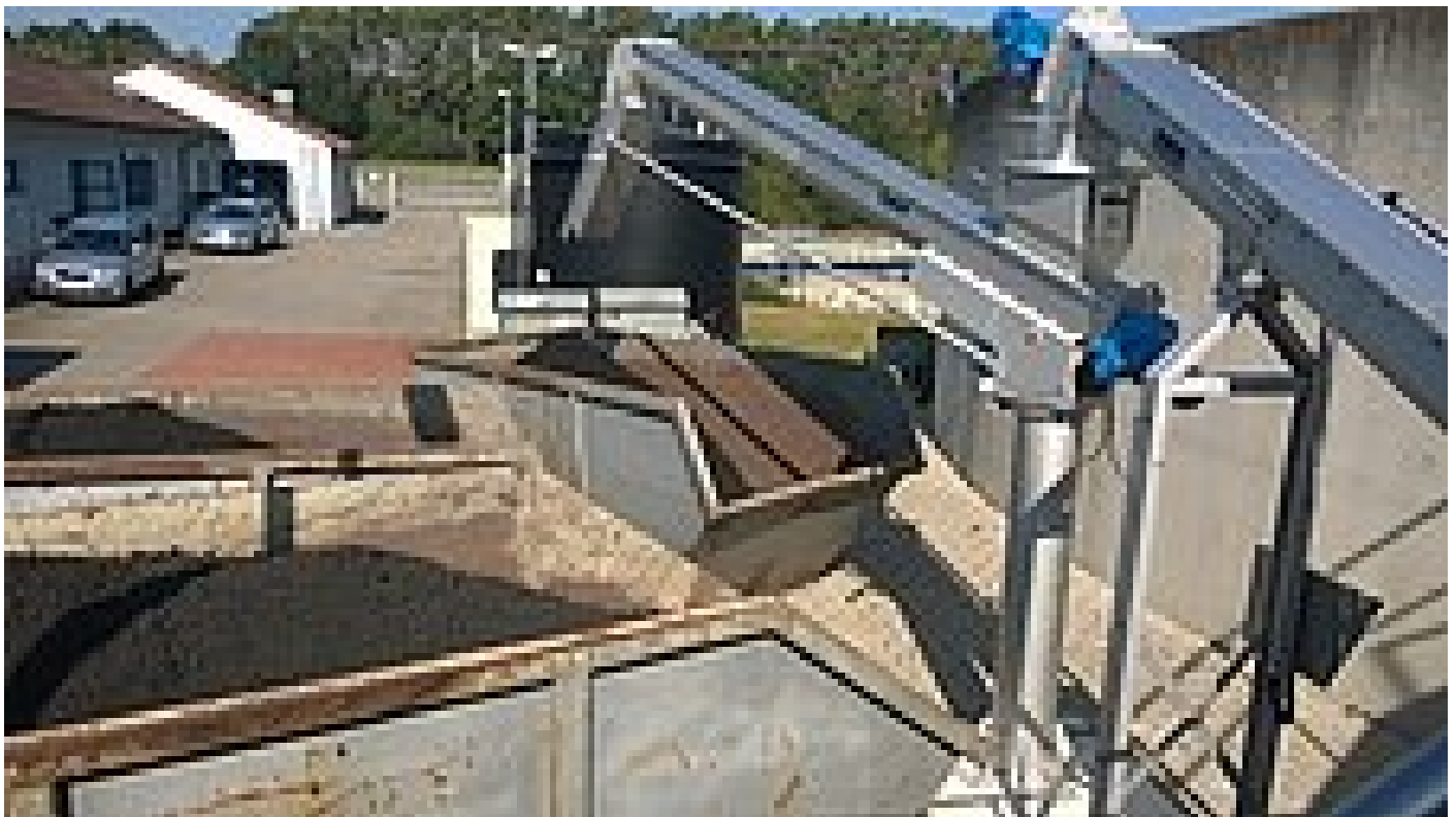
HUBER Screw Conveyor Ro8 T transporting dewatered sludge on STP Hausen. Freely rotating discharge system with an adjustable chute for easy, variable container feeding
