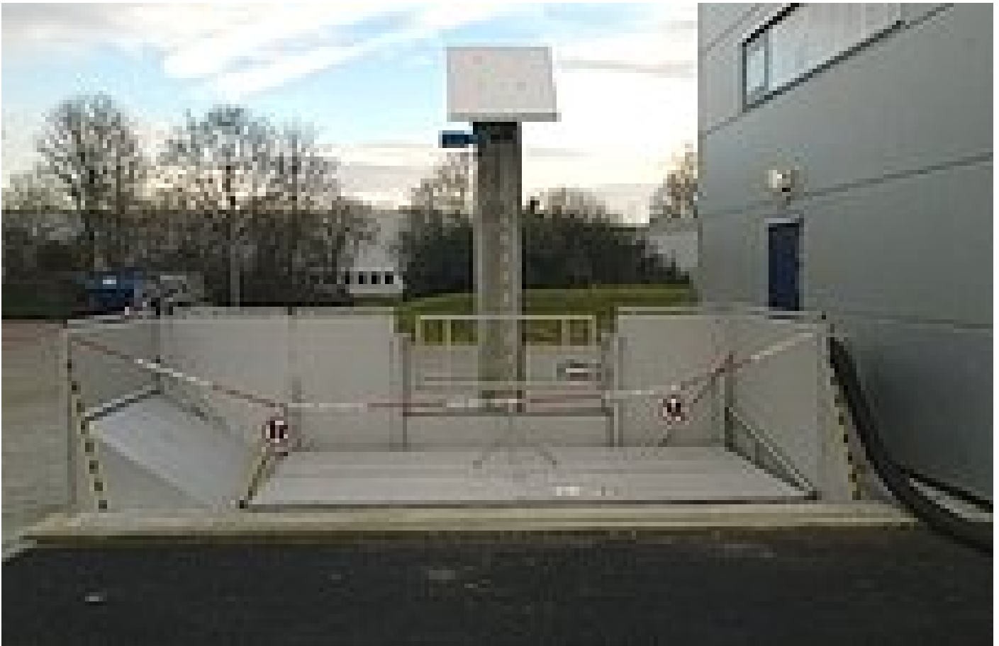
Grit treatment system RoSF5HW with automatic covering of the acceptance tank on STP Frankfurt Niederrad
