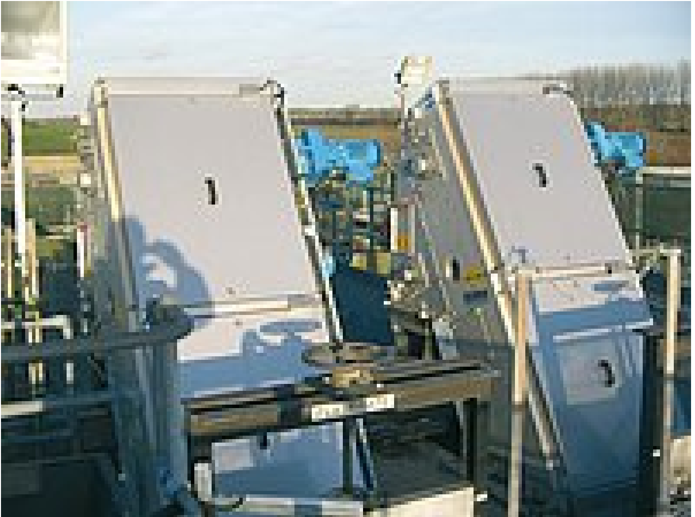
Sleaford, UK: Perforated band screens EscaMax® 4000
