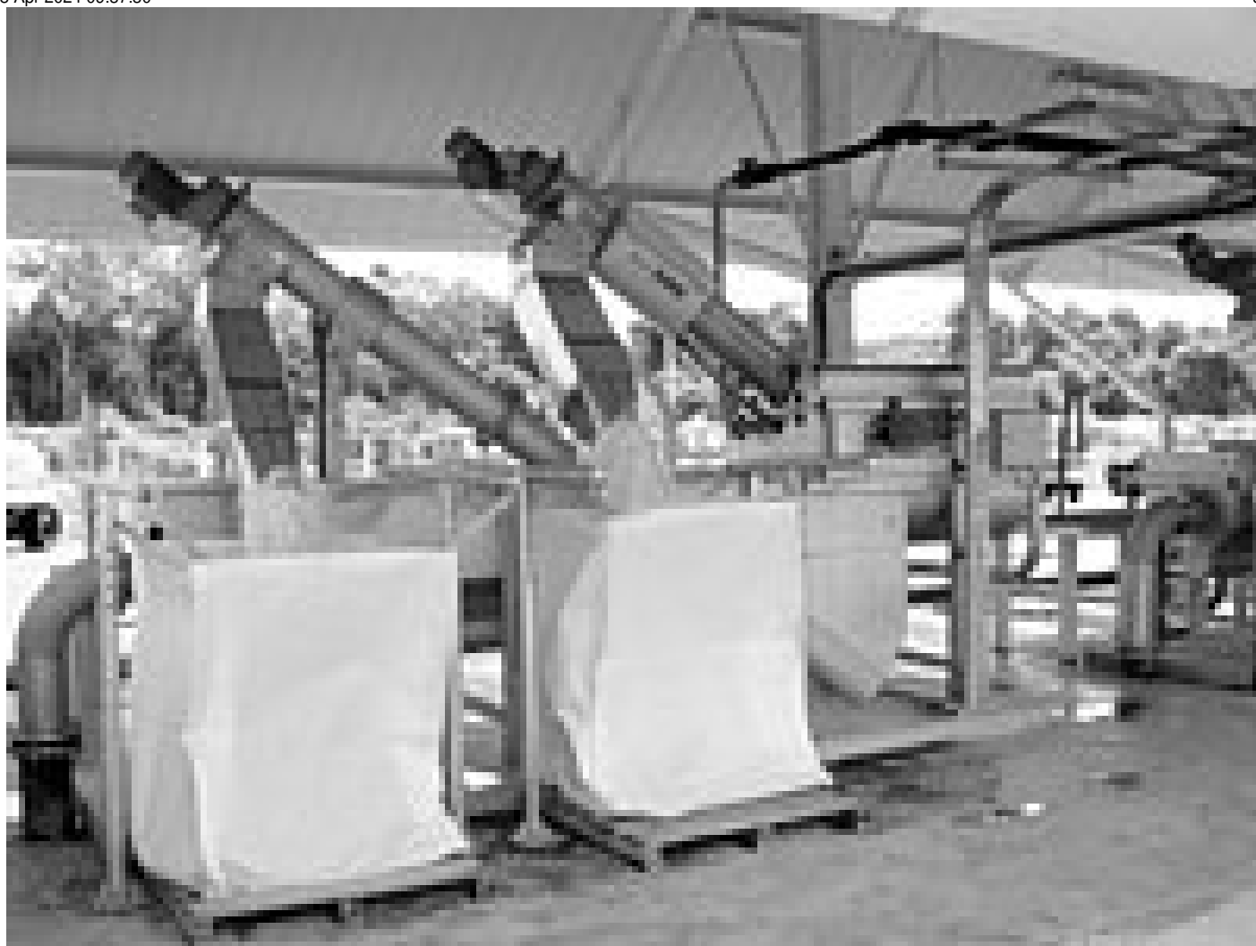
Complete mechanical preliminary treatment: removal of screenings and grit by the HUBER ROTAMAT® plant
