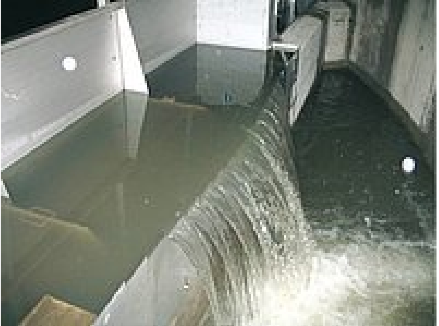
Sewage flowing through our RoK 2 screen and overflowing our measuring weir
