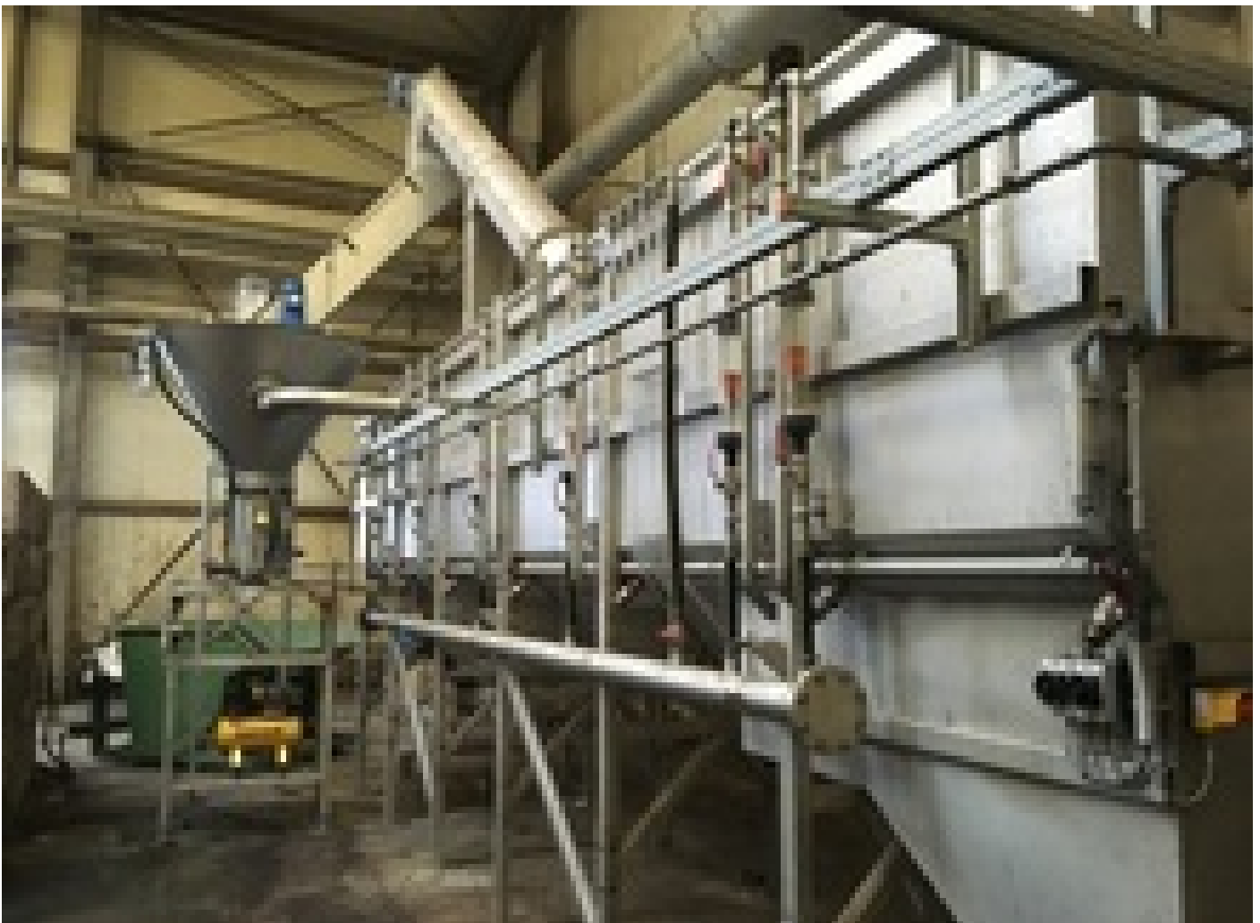
Fig. 1: HUBER Longitudinal Grit Trap ROTAMAT® Ro6 Bio (right) with downstream HUBER Grit Washer RoSF G4E (left)
