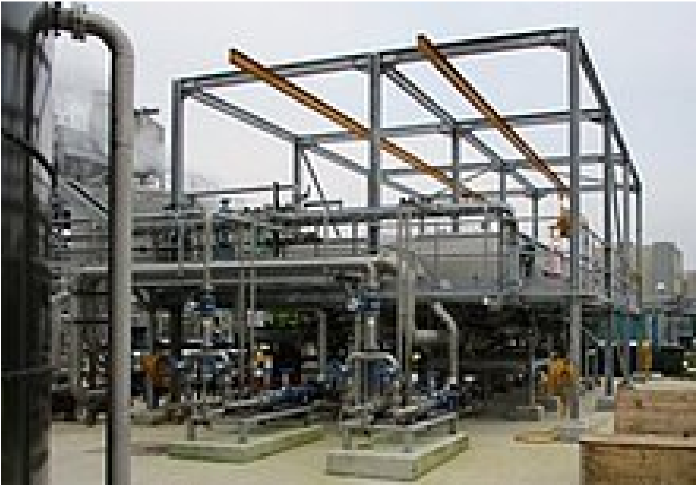
Figure 1 - DuPont Dissolved Air Flotation Plant installation with walkways
