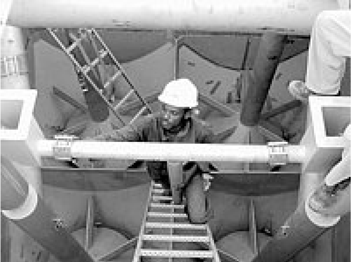
Interior of a Sandfilter
