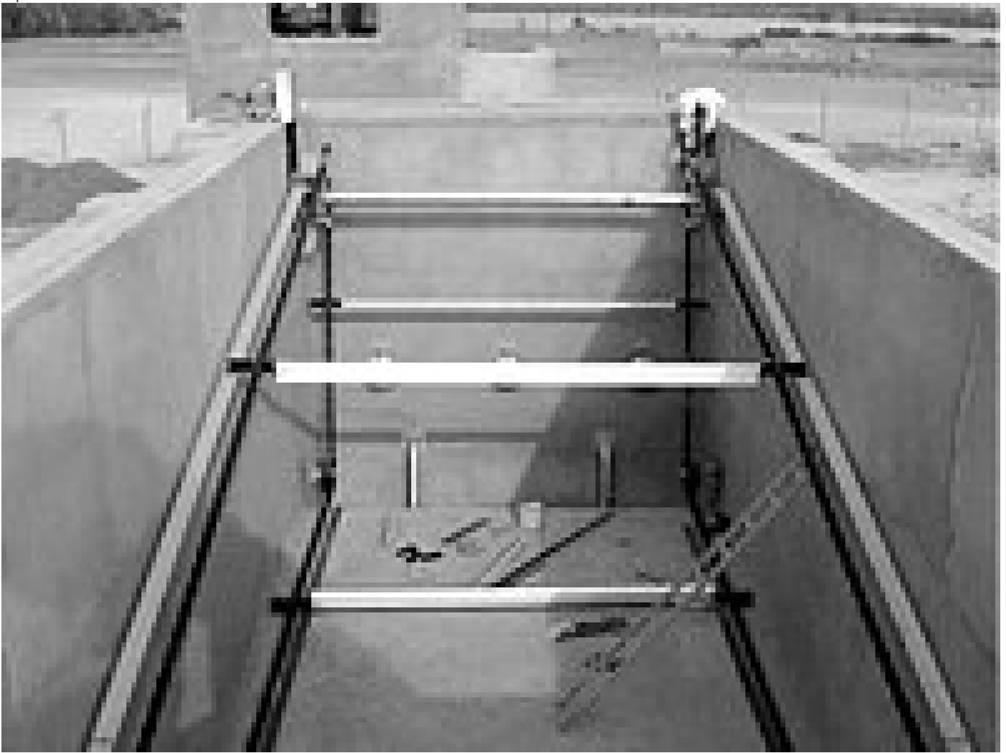
Sedimentation tank before start-up
