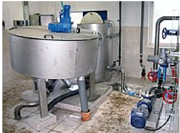
The latest RoS2S plant installed on WWTP Kolovraty, Prague in 2007
