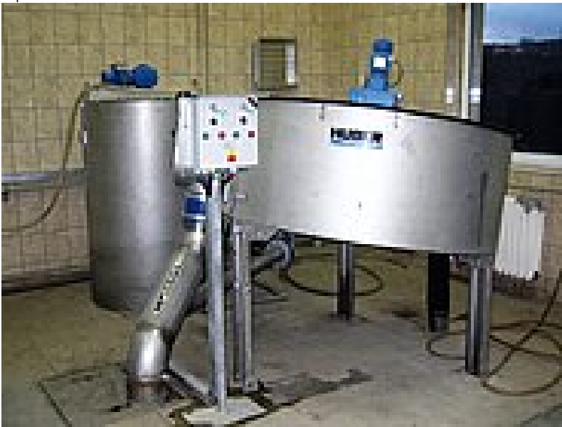
The RoS2S plant on WWTP Blansko designed in cooperation with main contractors KPRIA
