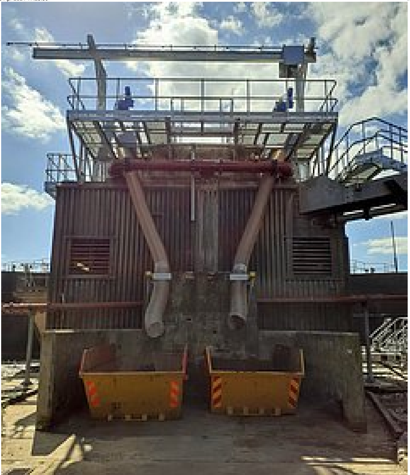
New screens and discharge chutes
